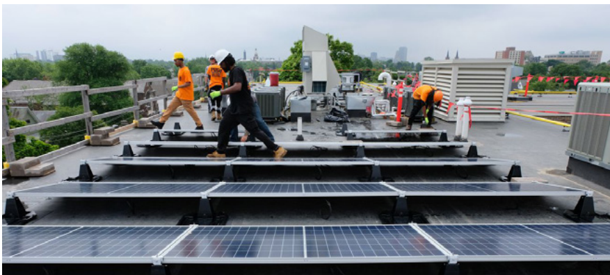
PUSH Buffalo Crew Installing Community-Owned Solar Array on School 77 Building (Photo from Curbed.com)
