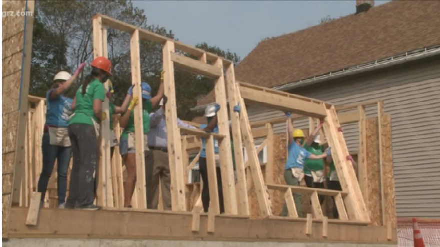
Habitat for Humanity Buffalo Constructing Home in Fruit Belt (Photo from WGRZ)
