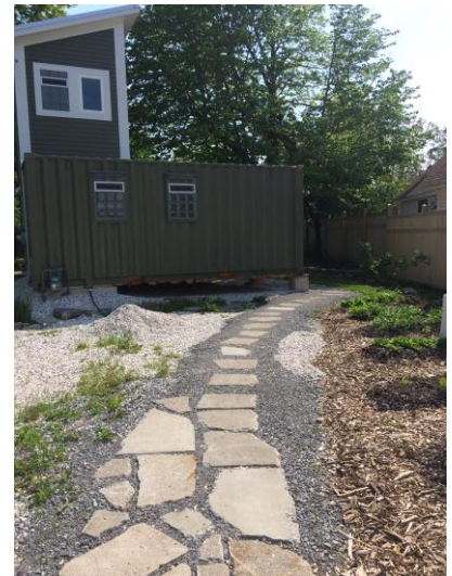
Nacho's hard work: broken-up "waste" concrete laid into an 8" deep bed of "quarter inch crusher."
